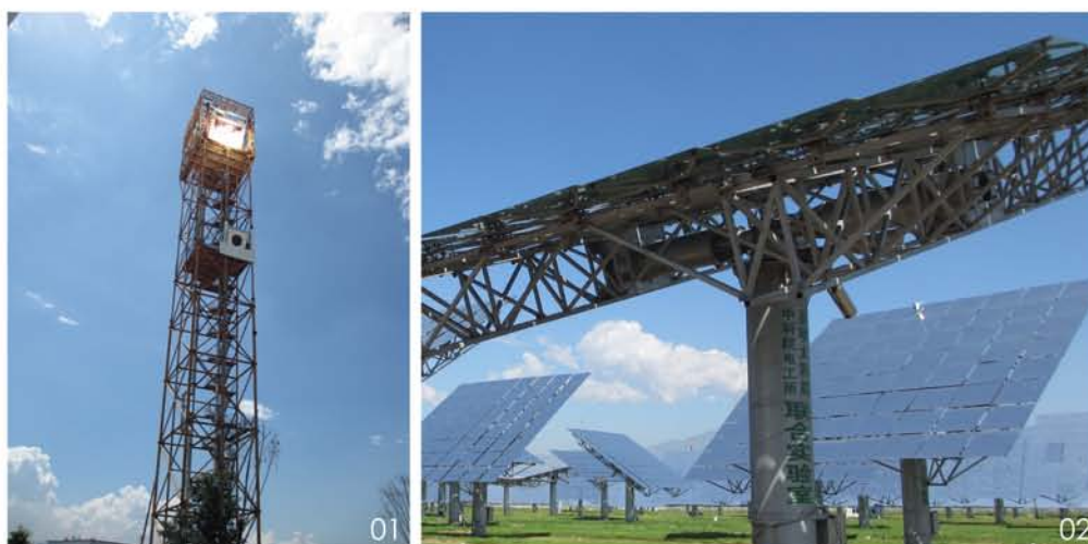
01/02 Beijing Badaling Solar Thermal Power Plant
